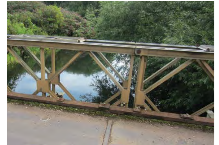
Access bridges require safety modification but otherwise provide excellent secure access to the site
