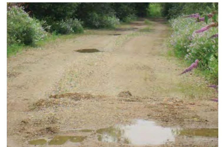
North haul road - to be regraded and locally repaired to form shared use link
